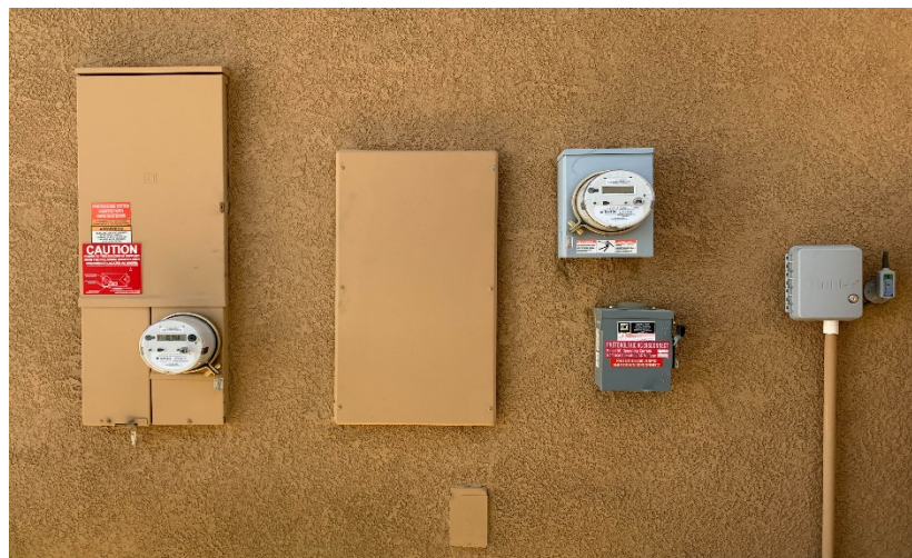
Electrical Set-up for a residential photovoltaic system – Photo by Juvoni Sterling
